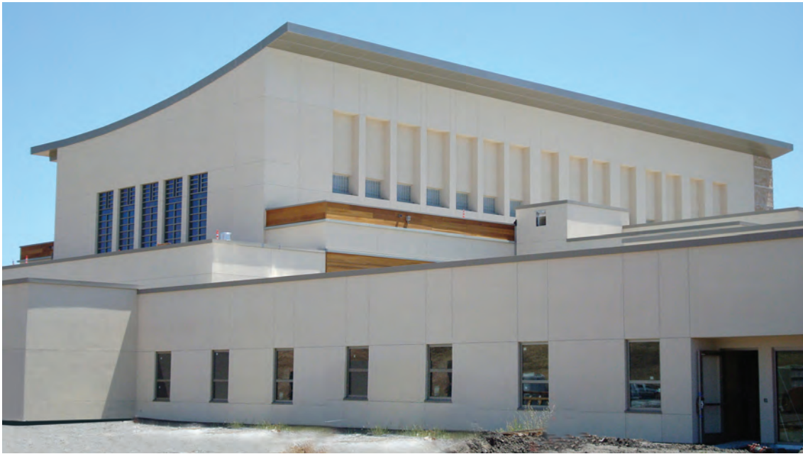
The Green Music Center under construction at Sonoma State University Rohnert Park, California
