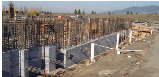
Managing the site's high water table required some clever design and construction.
