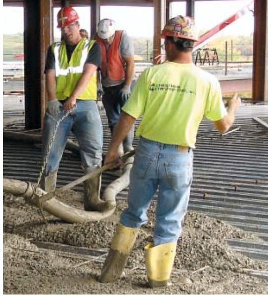
One of the nation's largest applications of synthetic macro fiber construction on steel composite decks, STRUX® 90/40 was used in place of welded wire mesh reinforcement.
