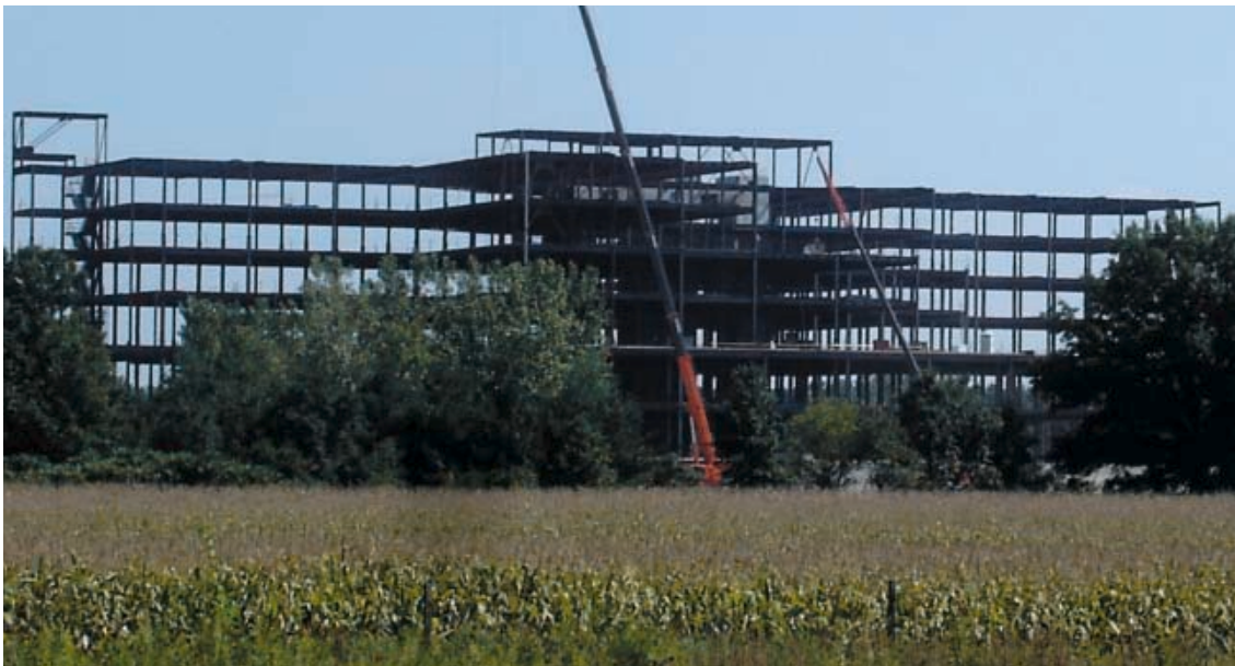
The Saint Joseph Regional Medical Center at Edison Lakes under construction. Mishawaka, Indiana.
