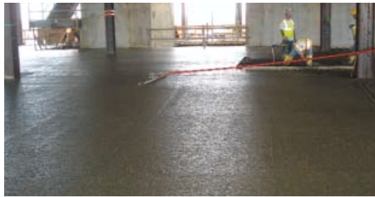
In addition to eliminating the time, cost and safety concerns associated with welded wire mesh reinforcement, STRUX placed and finished easily while minimizing cracking.
