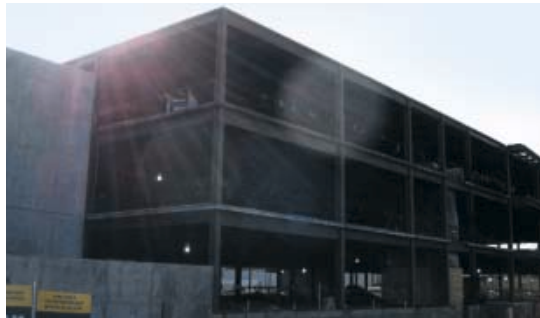
With new regulatory approvals, the combined facility was one of the first applications in the nation of STRUX® 90/40 synthetic macro fibers in elevated concrete and steel composite decks.
