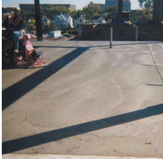
STRUX eliminated the need for welded wire mesh reinforcement and helped maximize crack control and durability.
