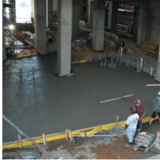
Workers finishing the slab near the main viewing tank. Using STRUX 90/40 synthetic fiber reinforcement to replace welded wire mesh for secondary reinforcement reduced safety hazards and helped to maintain the schedule, saving time and money.
