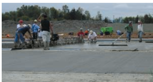
With no steel to trip over, the vibrating screed speeds the placement operation while STRUX helps provide high strength and tight crack control.
