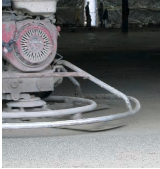
The use of STRUX 90/40 provided structural integrity to the concrete floor with no fibers visible on the surface.
