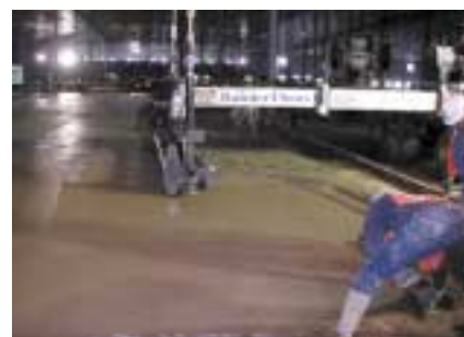
The use of Eclipse ® Floor enabled extended joint spacing in busy high-speed drive aisles and created a durable, low maintenance surface.
