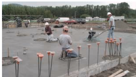
The use of Eclipse® Floor enabled extended joint spacing, saving time and maintenance costs
