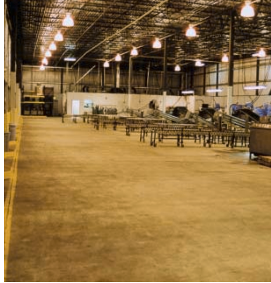
The plant's use as a cold storage facility required sloping floors, extended joint spacing, and an innovative solution to make it all work.
