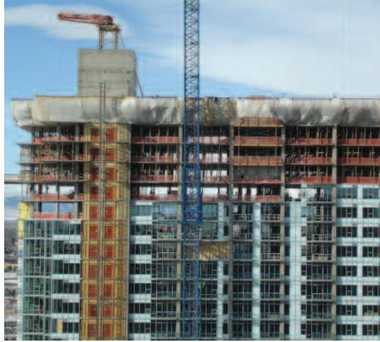
The high-rise contains two massive concrete cores with walls up to three-feet thick which were created using approximately 8,000 cubic yards of SCC and a new state-of-the-art admixture technology, Grace's ADVA® 408.
