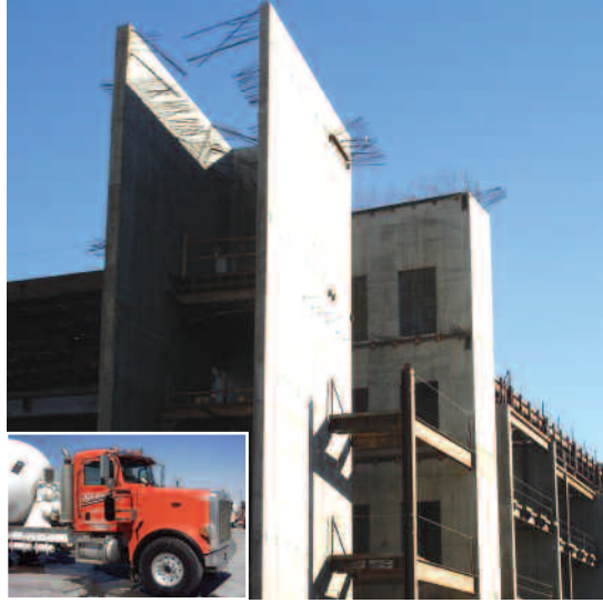
Nearly 2,000 cubic yards of highly flowable Self-Consolidating Concrete (SCC) with ADVA® 405 were poured to create the Center's strong structural walls – built to withstand seismic activity.
