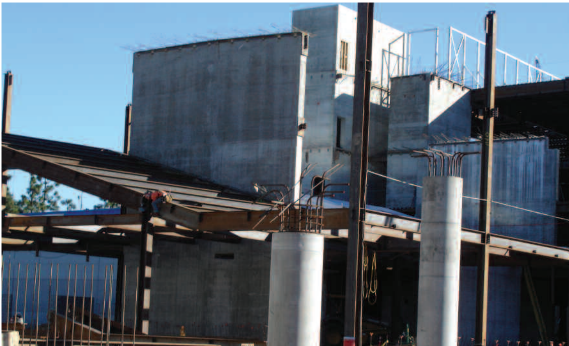
The Western University of Health Sciences Health Education Center under construction Ponoma, California
