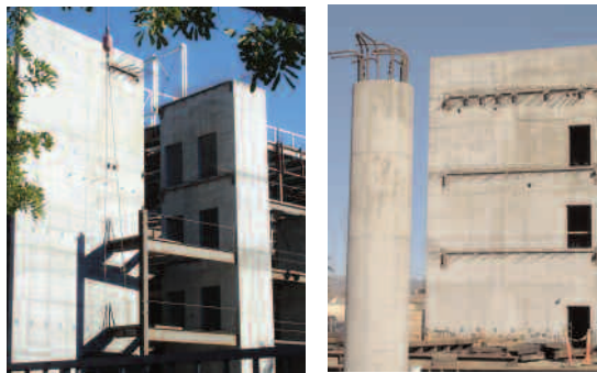
ADVA® 405 enabled the SCC mix to consolidate easily around extensive steel reinforcement within the formwork while still achieving the specified 6,000 psi compressive strength.
