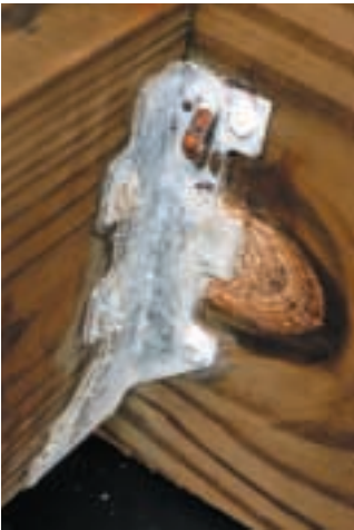
Galvanized joist hanger attached to ACQ wood, 7 months; wet conditions.
